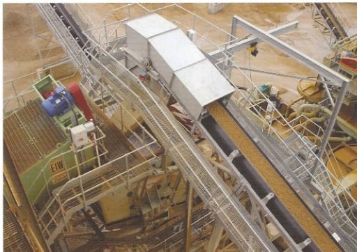
View showing the crushed material being returned to the second rinsing screen, with part of the Eagle Iron Works coarse material washer visible on the left
