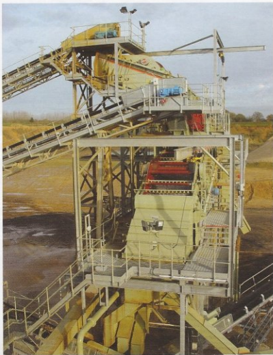
View of the washing plant showing the two Metso Ellivar 13 rinsing screens
