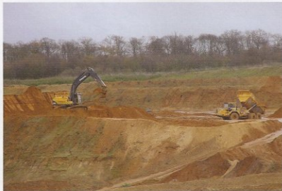
Careful blending of the sand and gravel is carried out at the face
