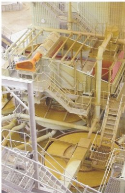
The computerized sand plant is capable of handling up to 600,000 tonnes per annum of -5\text{mm} feed to produce two main specification-controlled products
