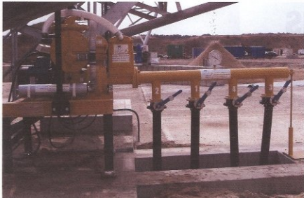
A moisture-reduction system for the drying of medium-grade sand stockpiles has been installed at Tarmac's Colchester Quarry
